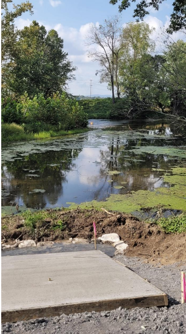
Figure 29. The boat launch site pad under construction in the foreground, with a young deer standing ankle deep in the North River in the background.
